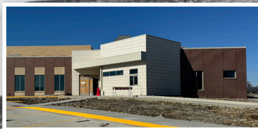
Construction progress on the new lab and clinic expansion as of November 2024.
